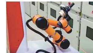
High-voltage distribution cabinet operation
